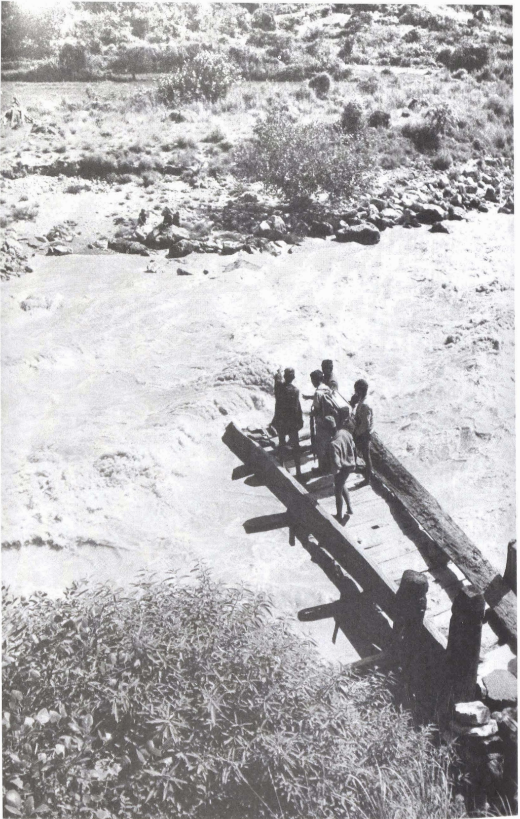
Fig. 81. A major washed-out cantilever bridge at Gum. On August 6, 1969, monsoon floodwaters destroyed all spans across the Mugu Karnali River, severing traffic between Humla District and the south for six weeks.
