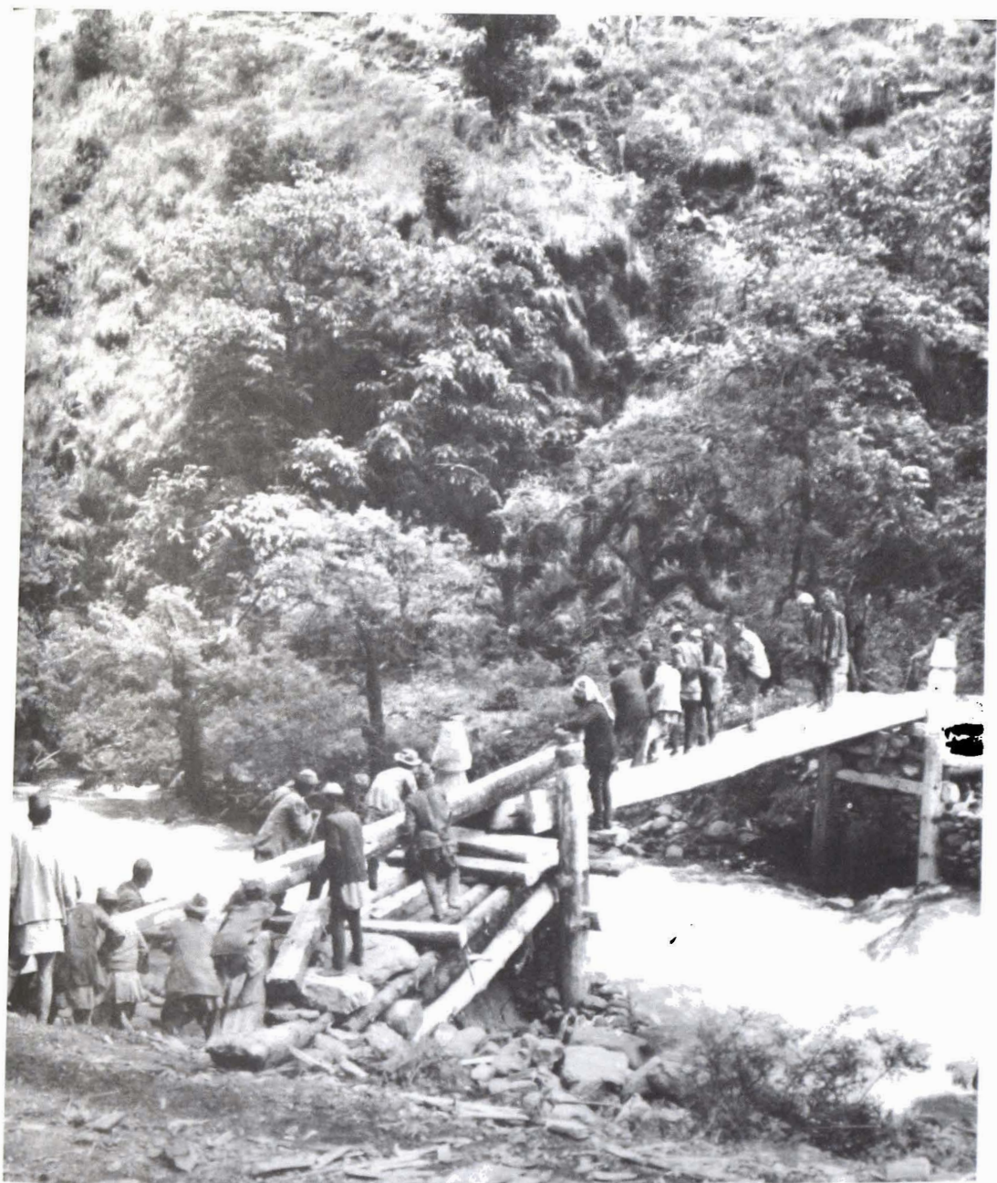
Fig. 94. Construction of a cantilever bridge in Chaudhabisa Dara. When completed, the bridge will permit access to the trail on the south-facing slope in the background, which becomes snow-free earlier in the spring.
